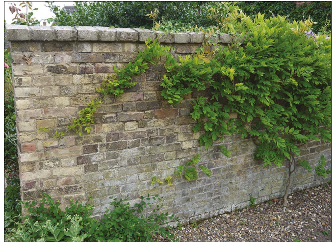
Figure 44: Lodge Close Wall.
